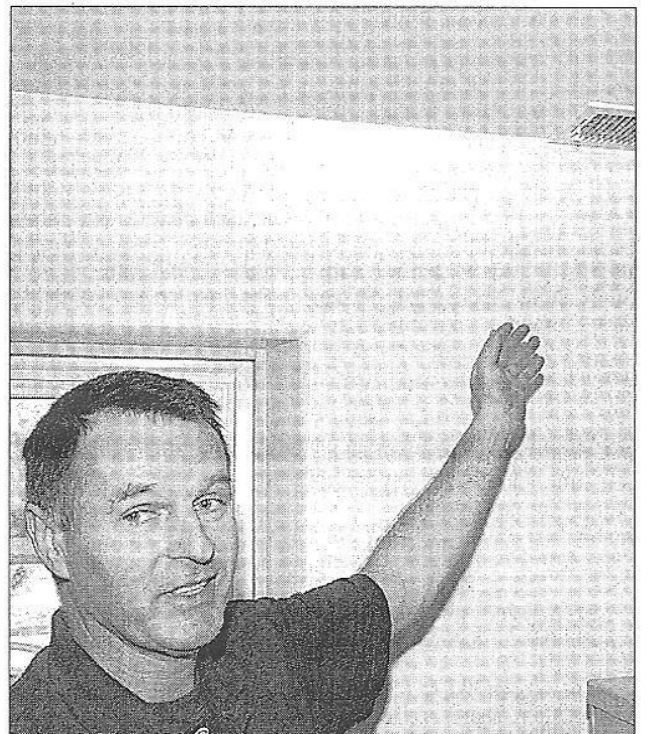
Alan Rushforth points out one of the solar vents that are installed in his home.
